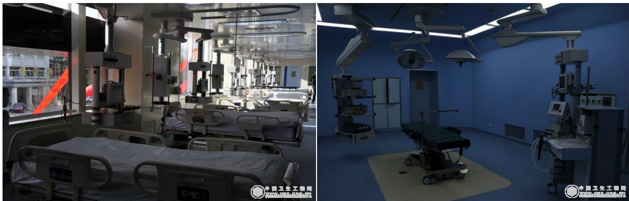
ICU ward and operating room in the new medical building at Navy General Hospital
